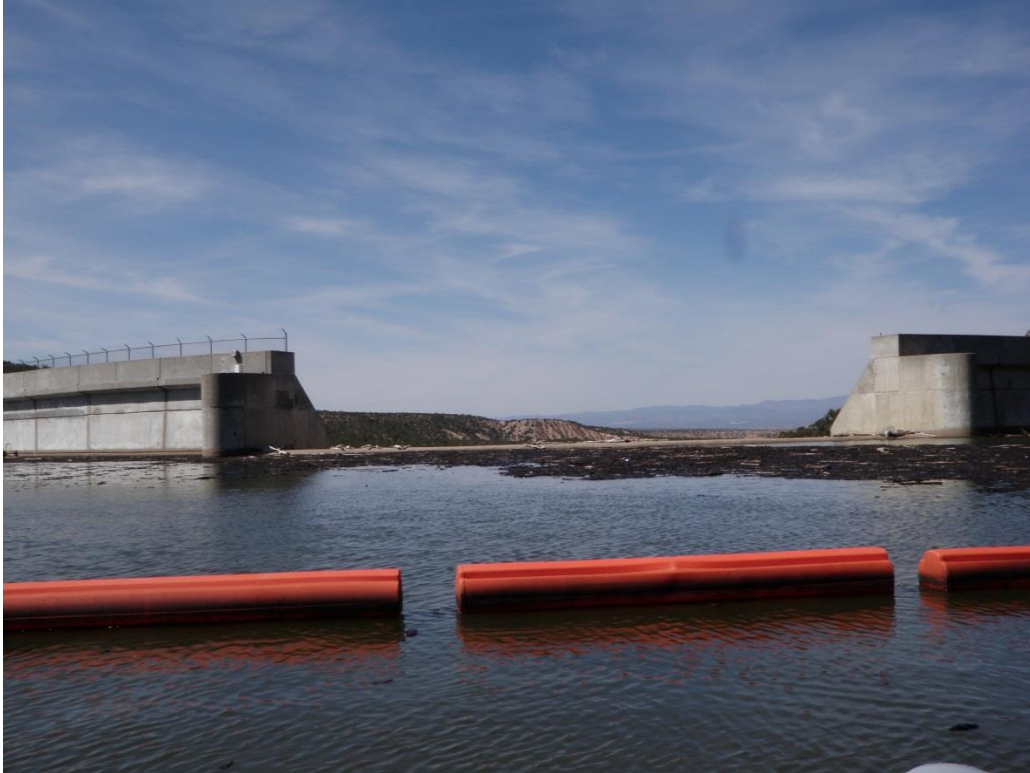
Figure 2 - Nambe Falls spillway, located in the concrete section of Nambe Falls Dam, with spillway crest elevation 6826.6 (NGVD29), March 2013.
